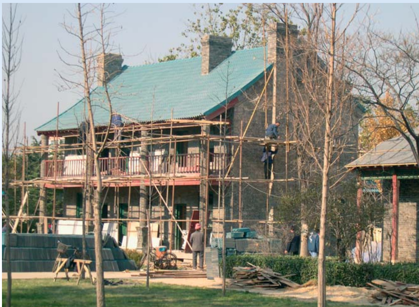
Restoring one of the original buildings of Zhoucun No 6 Middle School, November 2004.
