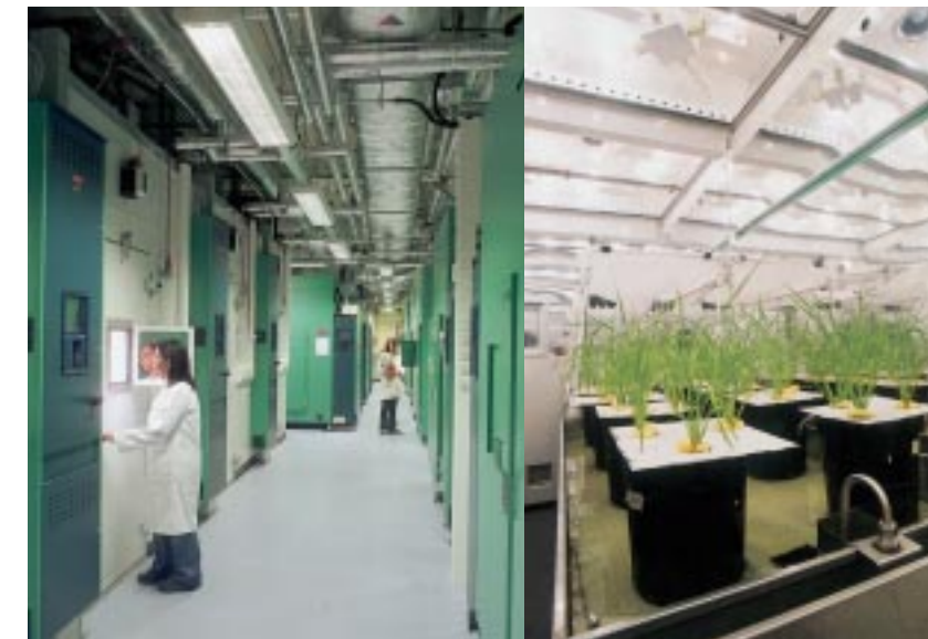
Left: Some of the 32 Controlled Environment Chambers. Right: Simulated 'paddy field' conditions for the growth of tropical rice in one of the chambers.
